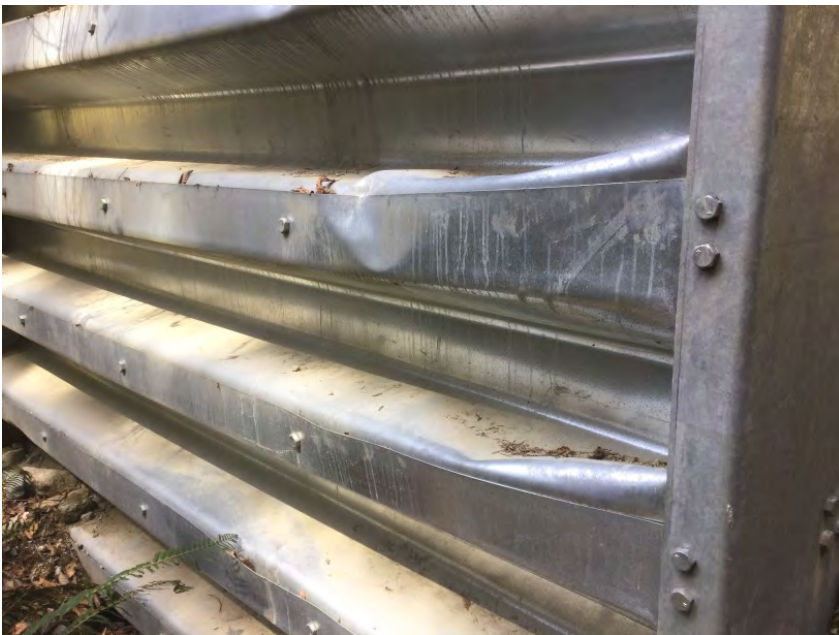
Minor damage noted at few location on bin wall - typical
