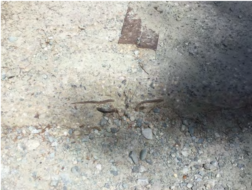
Damage to slabs noted at left bank
