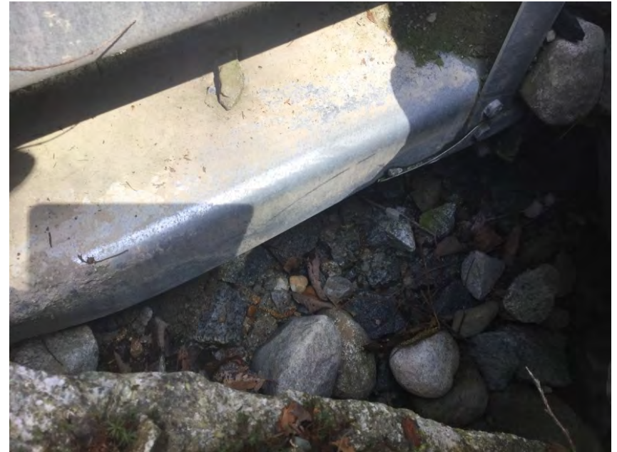
Material under upstream right abutment binwall eroding
